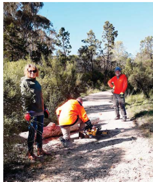
Annie Oakley, Robert Matthews and Greg Brown take a breather after cleaning up the debris along the repaired path.
